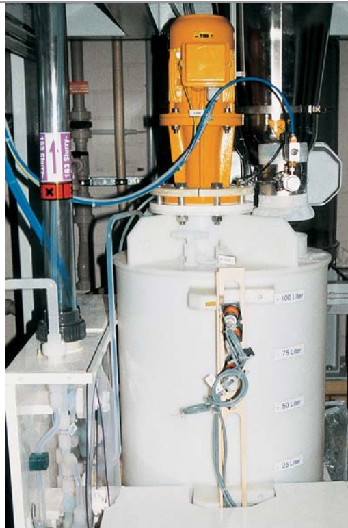
YTRON -Y installed on mating Flange of an Open Container Application: Suspension of Abrasive Polish
